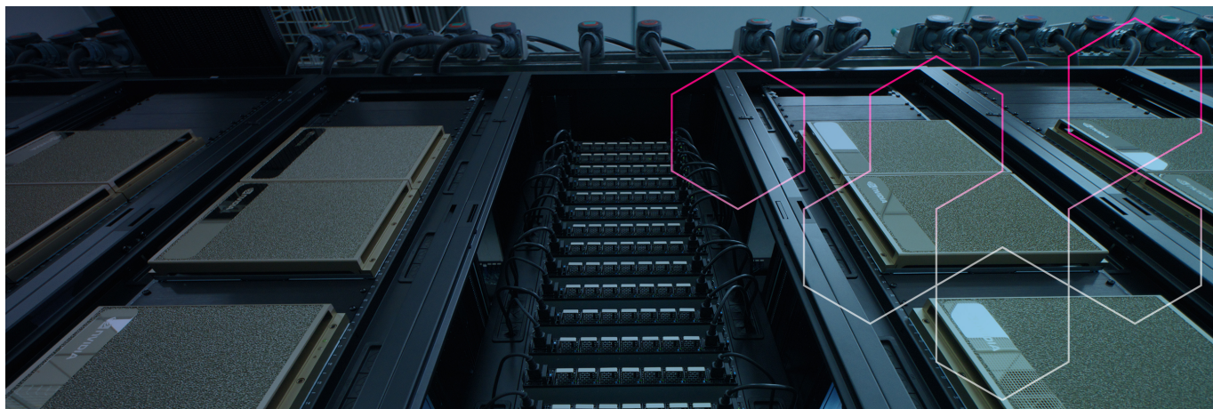
Figure 27. BioHive-2 is Recursion's new NVIDIA DGX SuperPOD AI supercomputer, powered by 63 DGX H100 systems with a total of 504 NVIDIA H100 Tensor Core GPUs interconnected by NVIDIA Quantum-2 InfiniBand networking. This NVIDIA-powered AI supercomputer results in over four times faster speeds than Recursion's original supercomputer, BioHive-1, in benchmark performance tests. Based on available data, BioHive-2 is the fastest supercomputer wholly owned and operated by any pharmaceutical company worldwide.
